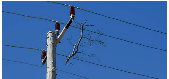
Fallen branches often cause temporary faults on powerlines
