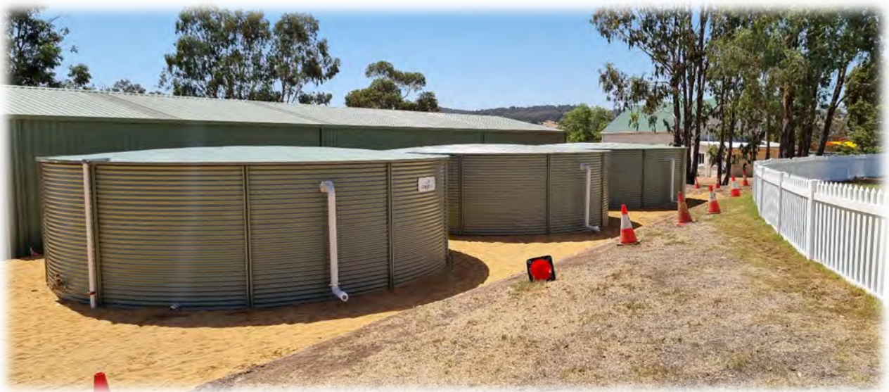
Collecting rain water run off from the machinery shed to re use at the public toilets
