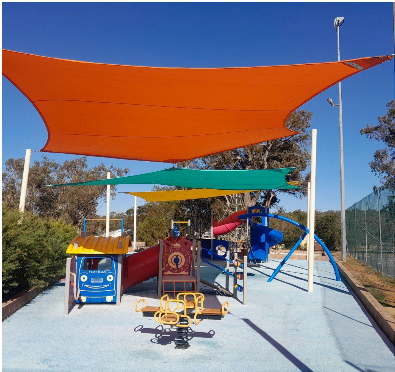
Figure above: Completion of the Community Centre children's play area shade sails install.
